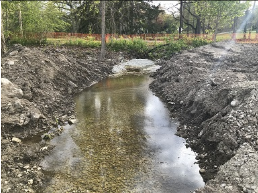
Stone channel on the site with pipe visible at the far end. Looking at Summer Street beyond construction fence.
