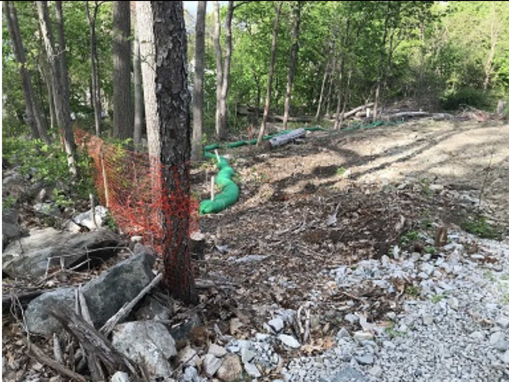
Entrance at Kilby Street construction fence is off site, property line stakes in upper center of photo. 5-12-21
