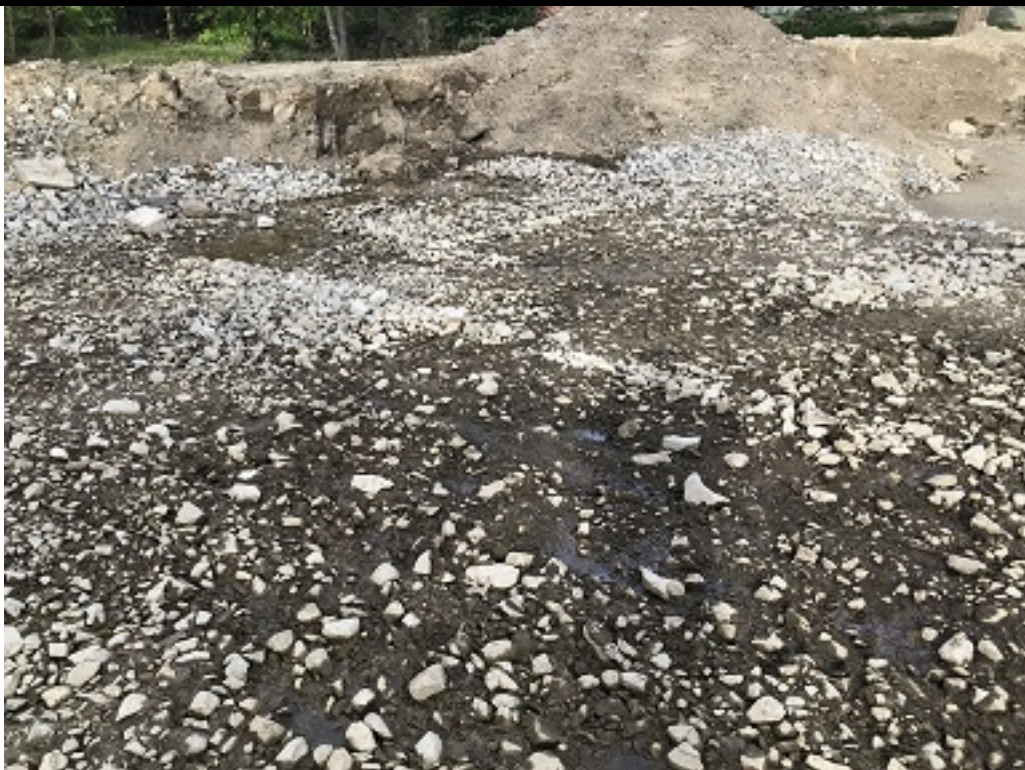
Approximate location of house pad at the time of my site visit water was visible in areas on the surface. 5-12-21
