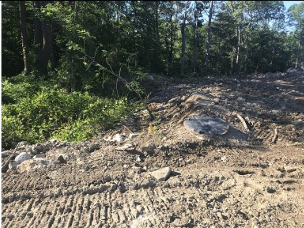
Looking South at a piece of exposed ledge behind the metal plate, it is unclear where the Tree Preservation Area is relative to this ledge but it would be to the right of the ledge in the photo based on prior estimations from available fencing. The stake is not identified.
