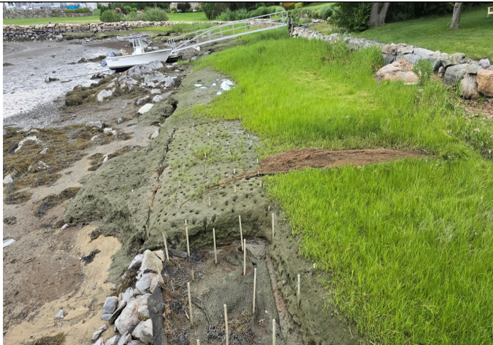
Salt marsh restoration area on northerly side of dock. Float damage fill has washed out.
