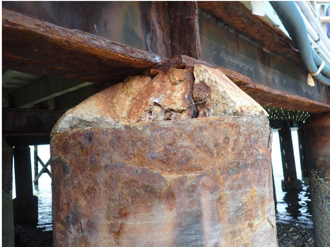
Photo 9 – Concrete-enchased H-pile to be repaired.
