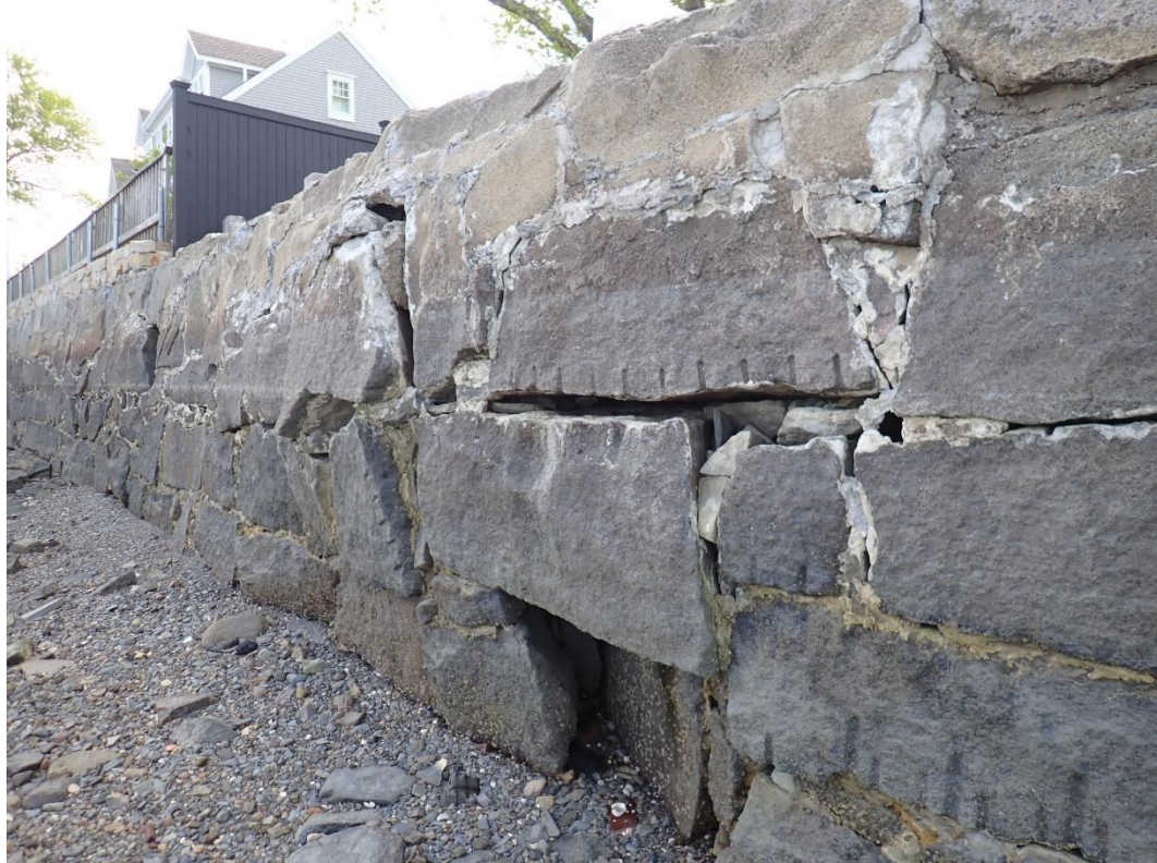
Photo 11 – Bulge in the masonry seawall at south end of 211 Downer Ave.
