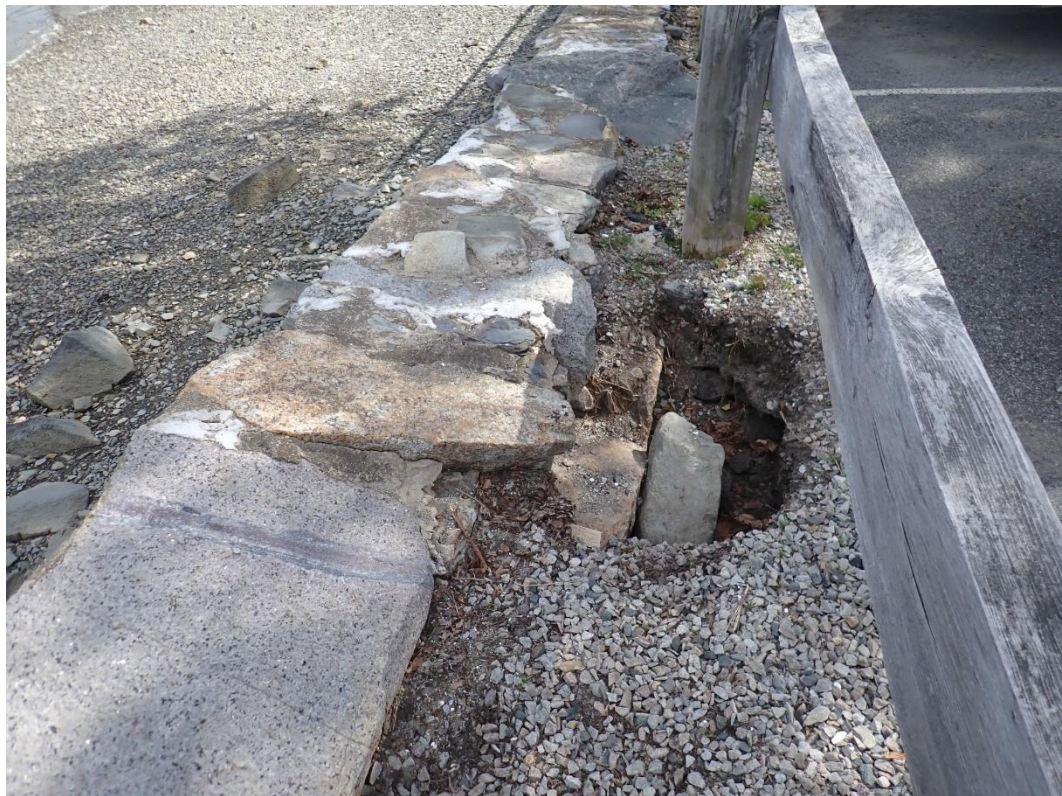
Photo 12 – Sinkhole behind masonry seawall at location of bulge.
